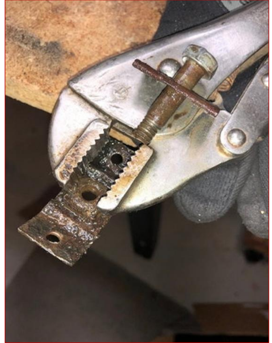
4) 2 Guys needed to lube, grab and loosen/tighten the rusted strap bolt. My plan is to clean, epoxy or drill out and screw a replacement underside nut plate retainer back in place later on...
