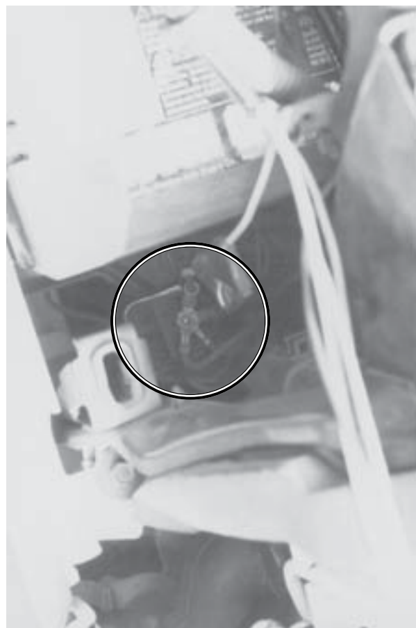
Power Terminal Connection (Adjacent to Battery)
