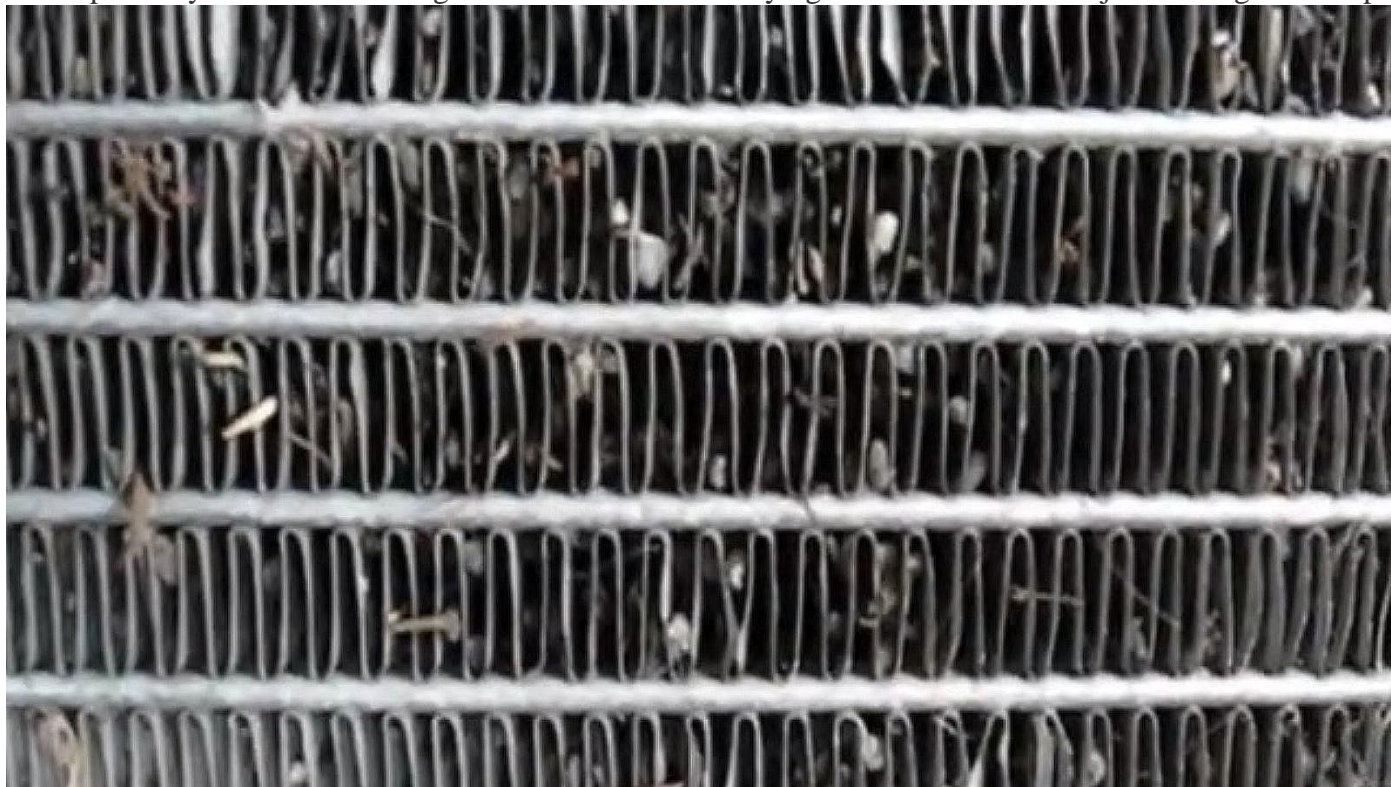
Figure 16. Close up of tiny stones embedded in A/C condenser.
